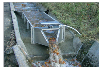
H-Flume for non-contact run-off measurement via ultrasonic sensors (Picture: Landfill Langenlonsheim, Germany)
