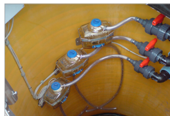
Measuring shaft with layered seepage water sampling and aliquot sampling (Picture: Landfill Profen, Germany)
