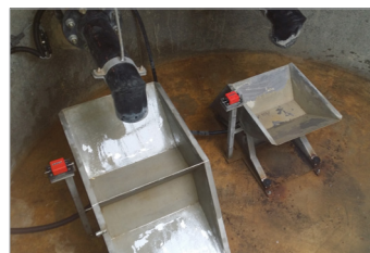
Service shaft with tipping counter volumes from 0.1-30 l (Picture: Landfill Seehausen, Germany)
